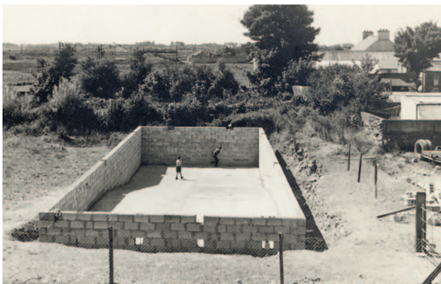
Ballyhaunis Swimming Pool under construction in the early 1970s, with a game of handball in progress.
